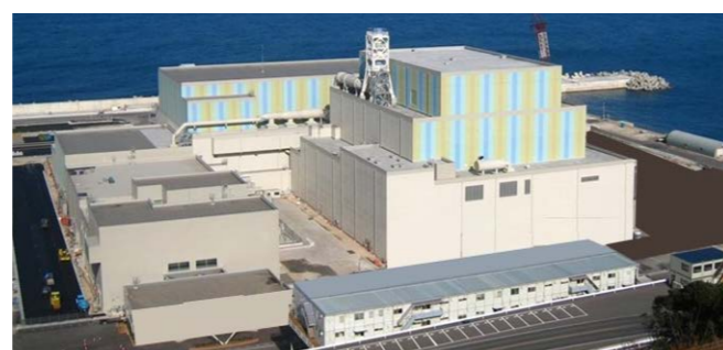
The Chugoku Electric Power Company, Inc.'s Shimane Nuclear Power Station Unit 3, under construction
