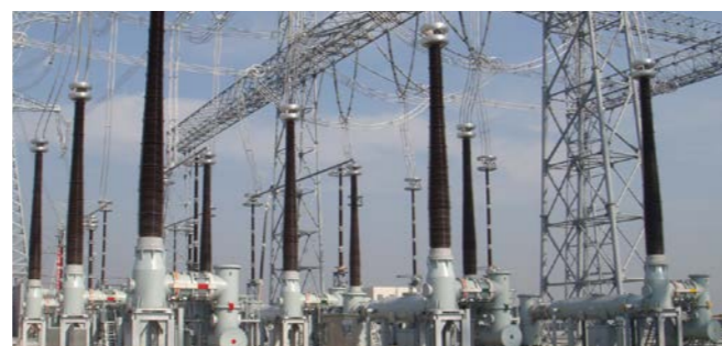
Ultra-high voltage gas insulated switchgear (UHV GIS)
