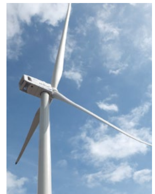
Fukashiba Wind Power Station in Kashima Port Hitachi Wind Power Ltd.
